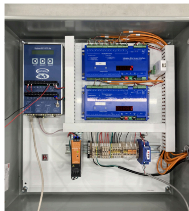
Remote access Vibrating Wire System
