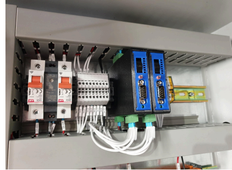
VibWire-301 in a PC Data Acquisition System
