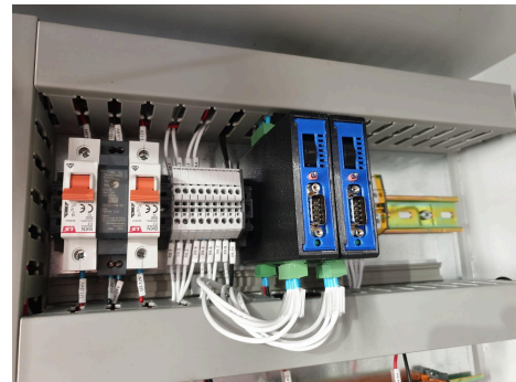
VibWire-301 in a PC Data Acquisition System
